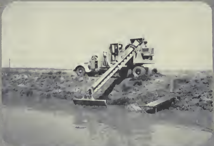
NEW MACHINE on the Tucuman project in New Mexico, scoops weeds out of hogwire trap. All photos are scenes from the new colored movie film "Weed Control on Irrigation Systems."
